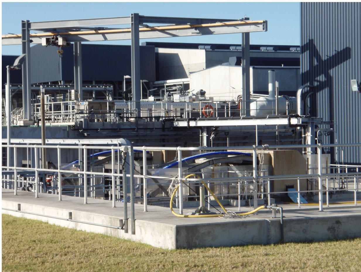
Overall view of VoR Drum Screens at Sydney Desal Plant
