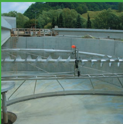
„in combination with submerged scrapers with a central drive unit and circular submerged effluent pipes“
