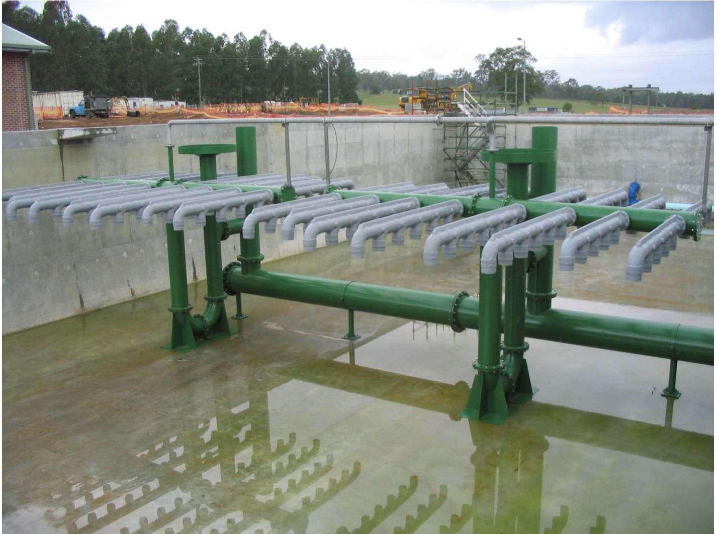
VoR – Gas Locked Siphon Decanters at Clarenza STP
