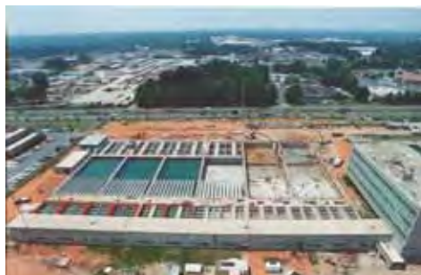
EXPANSION OF LAMELLA PLATE PACKS AND ZICKERT SLUDGE SCRAPERS INSTALLATION IN FRANKLIN, U.S.A.
