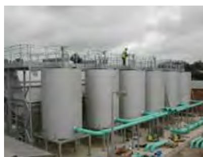
Installation of 6 flocc tanks of 19 m 2 each in the UK
