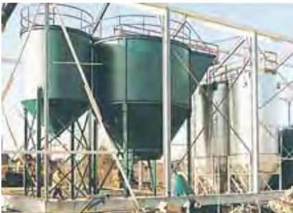
INSTALLATION OF A TREATMENT PLANT CONSISTING OF A SPECIAL PLATE SEPARATOR AND DYNASAND FILTERS.
