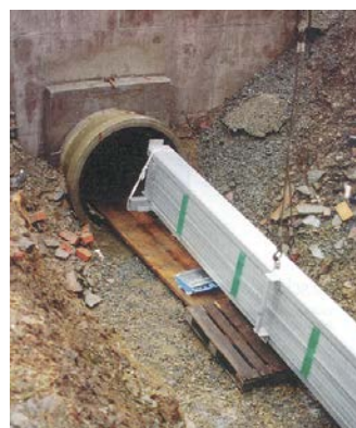
Screen admission through the outfall pipe
