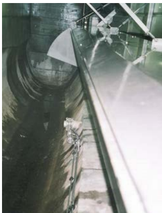
Contaminated bank area
