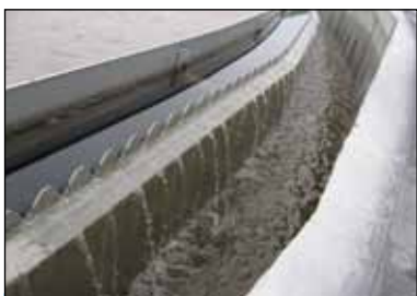
Concrete channel with: KD 16.17 Scum board KD 16.14 V-notch weir
