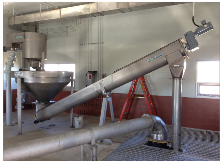
Installed GritCup / SpiraSnail system protecting downstream processes
