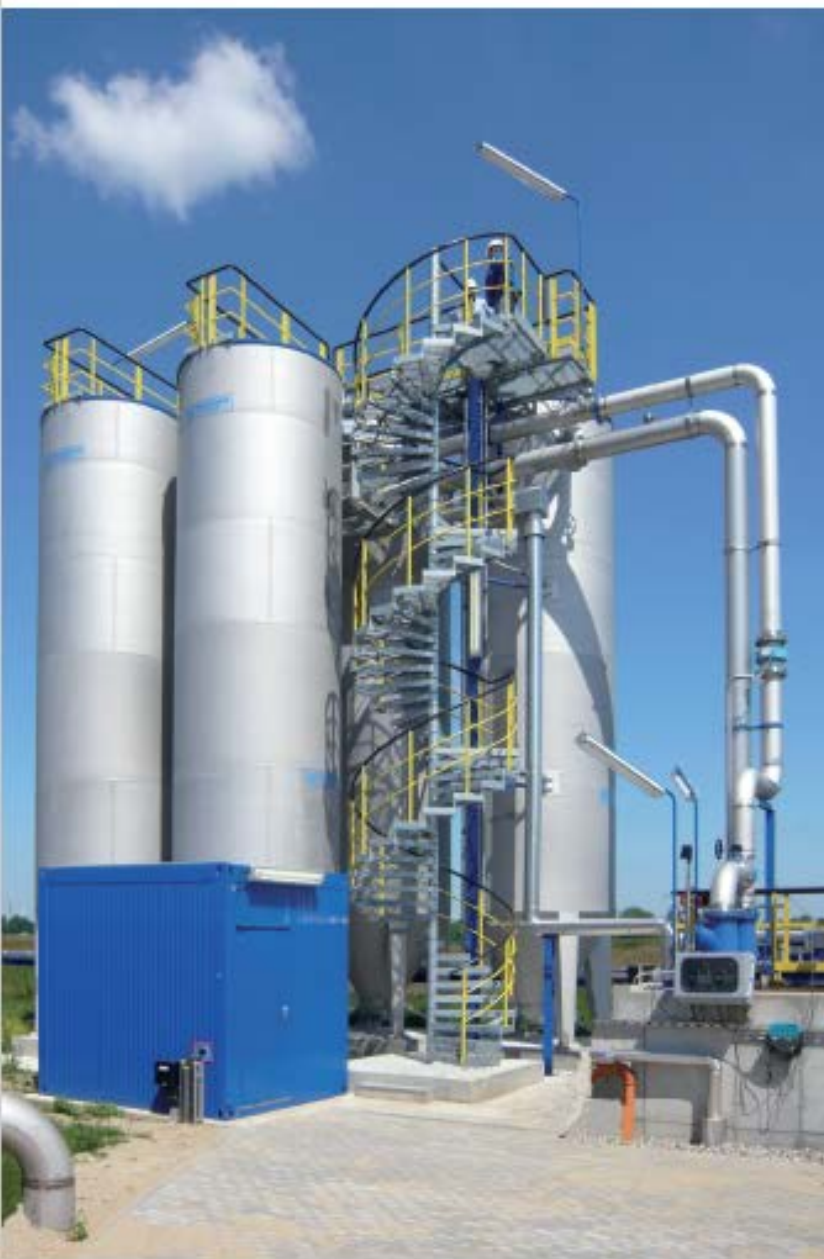
Nitrogen reduction with DynaSand Deni at Yara Brunsbüttel GmbH, Germany
