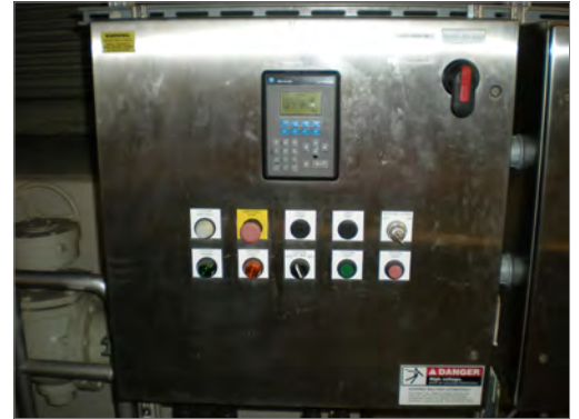
Control Panel with HMI
